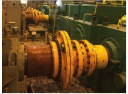
Shear pin gear couplings in steel mill
